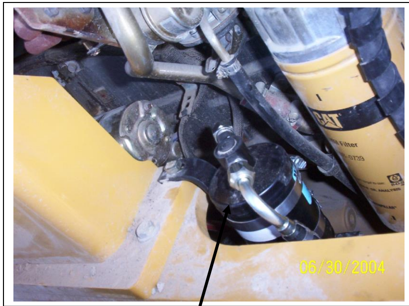
Receiver drier installed
